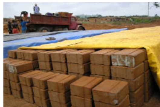
Fig. 3: Stacking and curing of interlocking blocks. Source: Field survey (2007), Obasanjo low-cost housing estate, Ado-Ekiti
