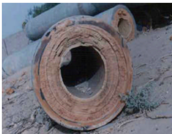
Fig. 1: Conducts water supply state in Oued R'hir valley
