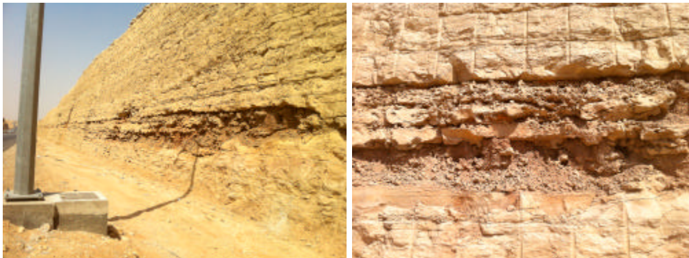
Fig. 1: The location of studied samples showing Cross-section of limestone rocks with strip of soil (Jubaila Formation)
