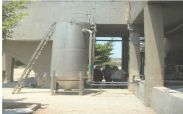
Fig. 2: The DynaSand unit located in Fostat water plant, Cairo, Egypt
