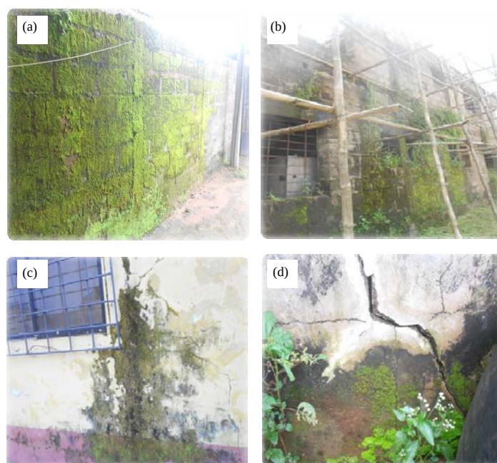
Fig. 9(a-d): Deteriorative effects of biological growth on walls, (a) Fence wall exposed to rain, (b) A building under construction, (c) Biodeterioration of wall paint and (d) Crack due to biodeterioration
