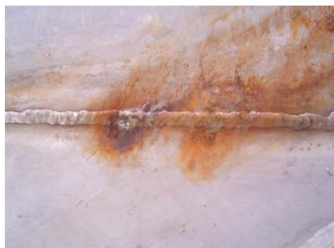
Fig. 1: Corrosion in vessel, around the fillet weld
