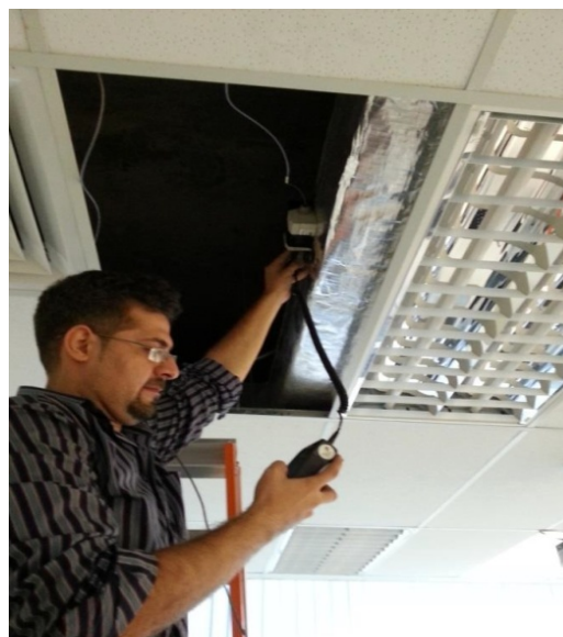
Fig. 6: Temperature and humidity measurement of supply air in main duct of FCU
