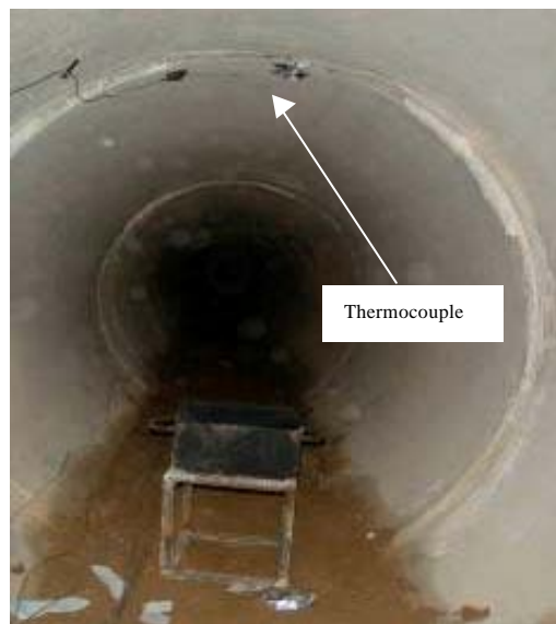
Fig. 2: Thermocouples arranged at the vault in the test
