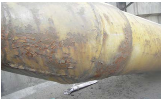
Fig. 5: Rusty spots on the outer surface of guide pipe
