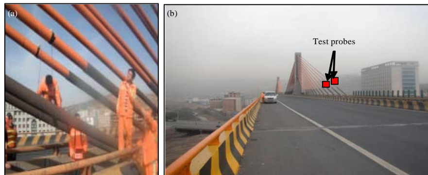
Fig. 2(a-b): Cable force test (a) Cable force measurement and (b) Layout of test probes
