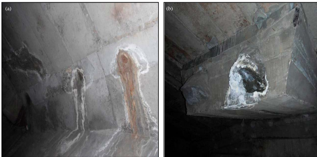
Fig. 8(a-b): Damage of girders (a) Girder roof and (b) Water erosion in the anchorage of girder roof
