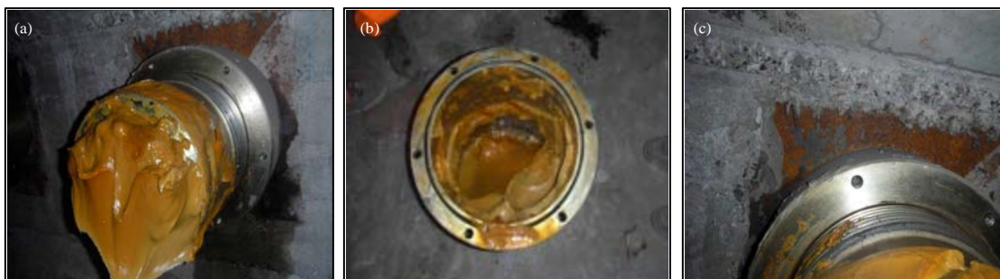
Fig. 6(a-c): Typical damage of anchorage systems (a) Ends of the anchorage, (b) End cap and (c) Corrosion of the bearing plates
