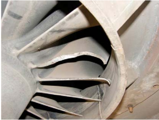
Fig. 1: Picture of blade failure
