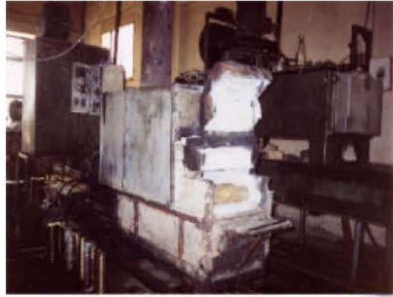
Fig. 9: The reheating furnace
