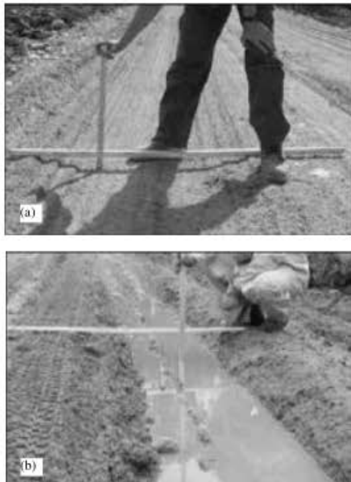
Fig. 3: Deformation classifying on rural road surface (a) shallow wheel ruts and (b) deep wheel ruts
