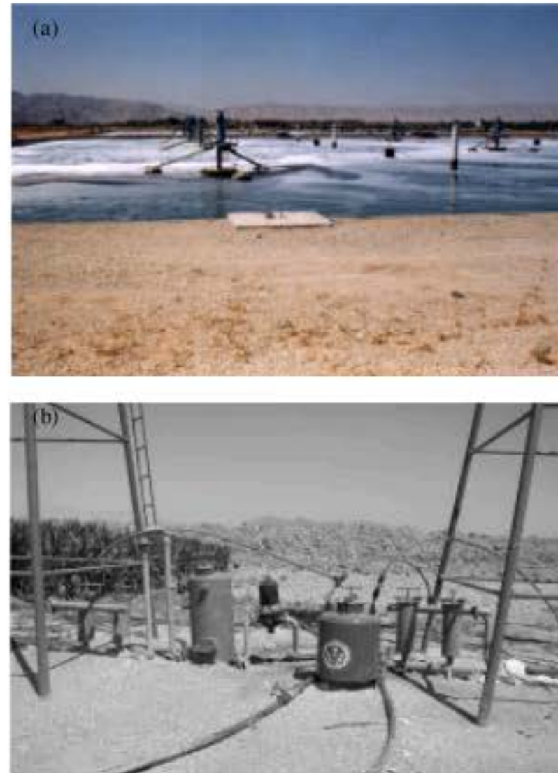
Fig. 1: (a) The sewage treatment site and (b) the filtration systems
