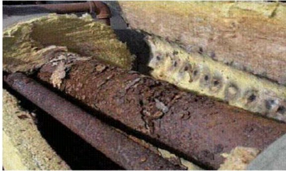
Fig. 1: Pipeline damaged by external corrosion
