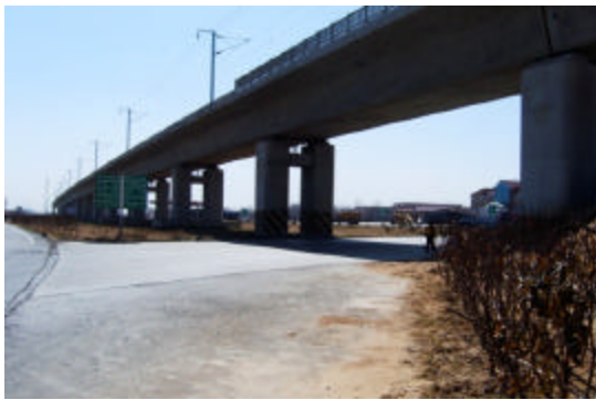
Fig. 2: Viaduct of passenger railway crossed the west of Xinzheng rest area at the entrance ramp
