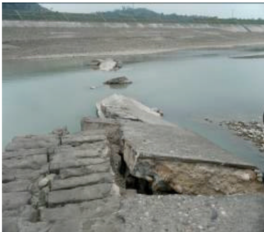
Fig. 2: Spur dyke water damage photos on xiaomitan
