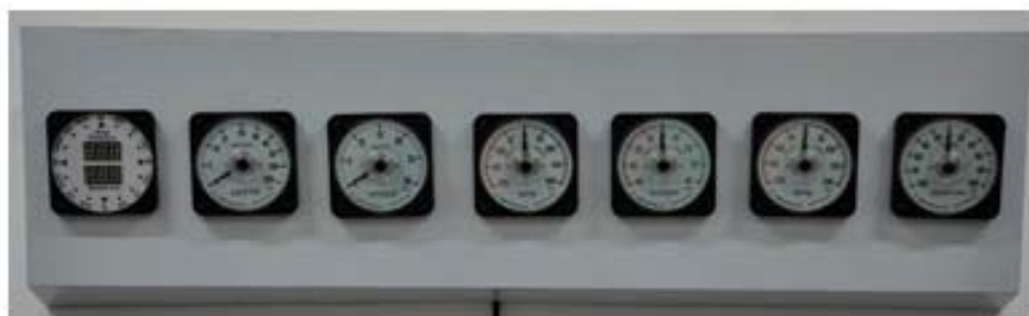
Fig. 5: The physical picture of instrument panel
