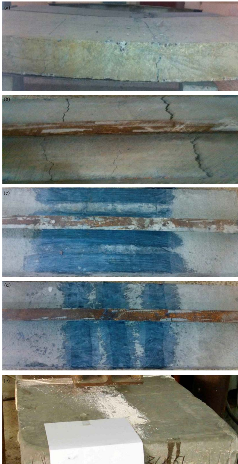
Fig. 3(a-e): Cracks generated and treatment in concrete deck, (a) Deck's cracks (Side), (b) Deck's cracks (Top), (c) Longitudinal FRP strip, (d) Transverse FRP strip and (e) Epoxy resin injection
