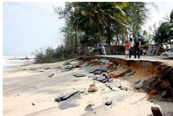
Fig. 1: Erosion occurs at the north side of the runway platform of Sultan Mahmud Airport, Kuala Terengganu
