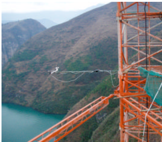
Fig. 2: Anemometer installed at 90 m above the arch springing
