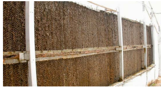
Fig. 1: Evaporative cooling, view of the pad end
