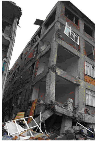
Fig. 1: Beam-column connection failure, Izmit, Turkey, 1999 earthquake
