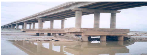
Fig. 1: Severe scour around the Kahank bridge piers in Khuzestan province
