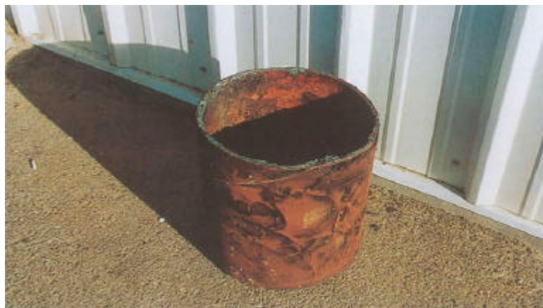
Fig. 2: Corrosion of well casing due to high salt concentration of groundwater
